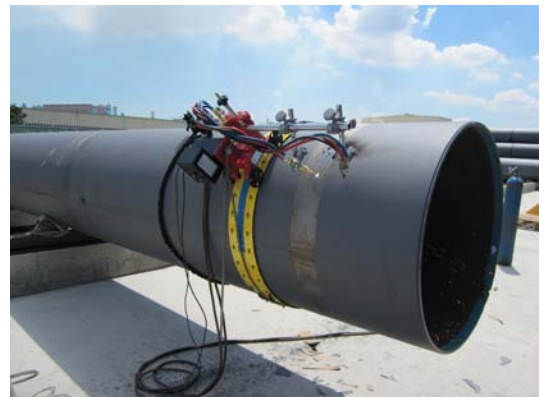
Oxyacetylene cutting, V-type of bevel Pipe size dia 1067mm, wall thickness 14mm
